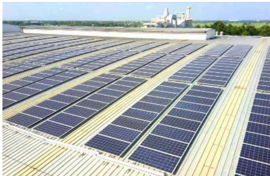
SOLAR ROOFTOP 2 Projects Chok Chai, Nakhon Ratchasima
