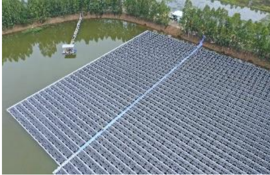
FLOATING SOLAR 1 Project Chok Chai, Nakhon Ratchasima
