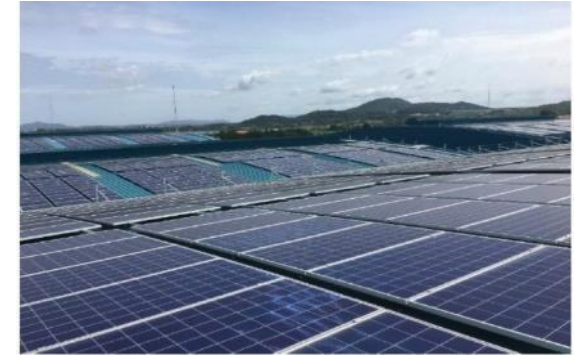
SOLAR ROOFTOP 1 Project (Extension) , Sriracha, Chonburi
