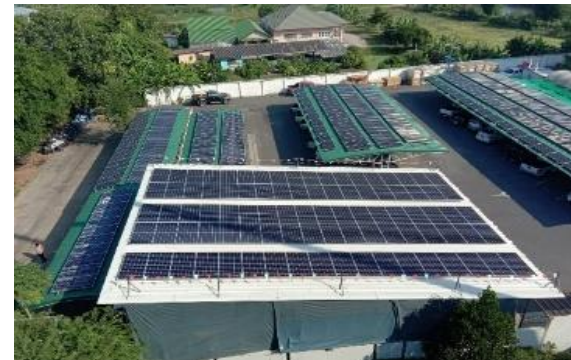
SOLAR ROOFTOP 3 Project Mueng, Samut Sakhon
