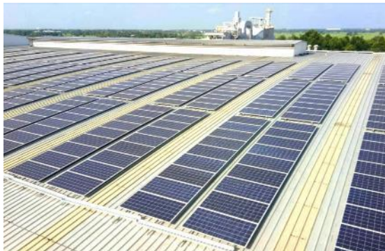
SOLAR ROOFTOP 2 Projects Chok Chai, Nakhon Ratchasima
