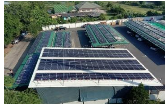
SOLAR ROOFTOP 3 Project Mueng, Samut Sakhon
