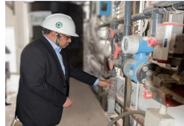
Md. Tajul Islam (Minister of Local Government and Rural Development) visited MSW KK powerplant at 16 Feb 2019
